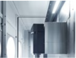
LED lighting in the working area.
