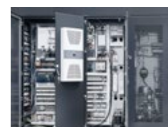
Climatized electric cabinet with easy access.
